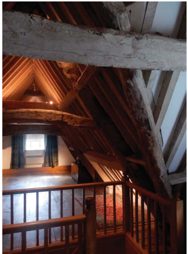
The attic, showing a few of the sturdy beams that have supported the house for more than 400 years.
